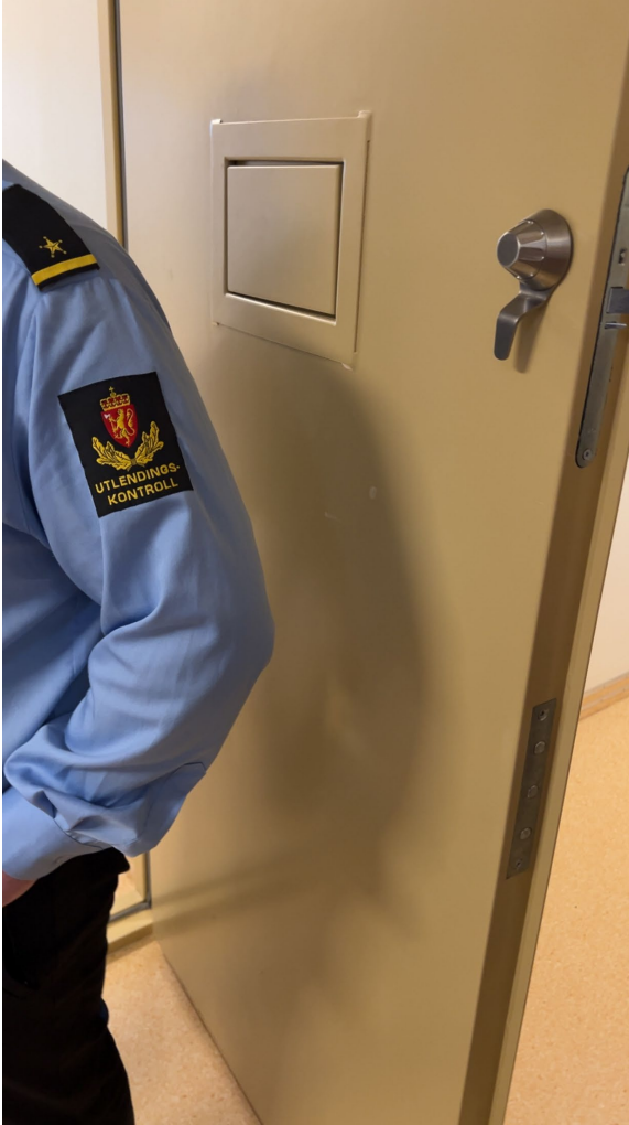
Cell door with newly installed cell lock
